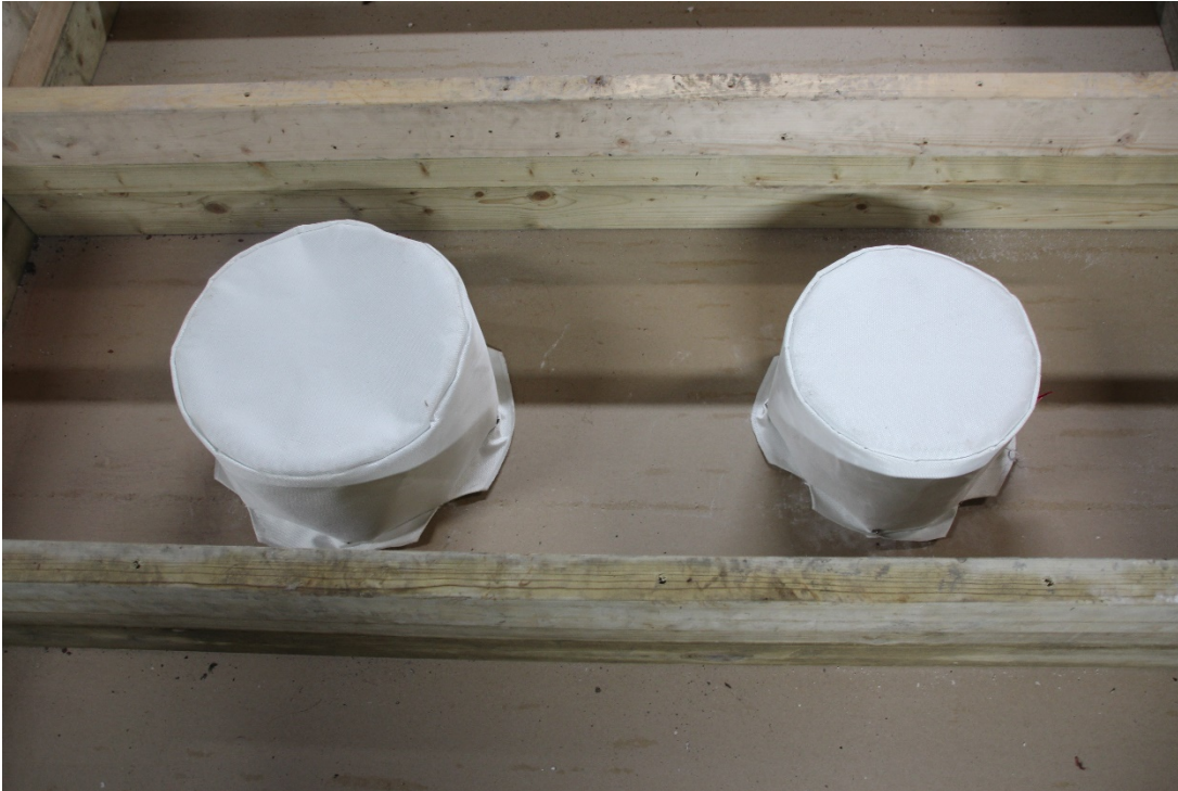
Photo 3 – Before test on unexposed side to show location of Hoody fireproof acoustic covers. This is before the 18mm OSB board was fitted over the top of the joists
